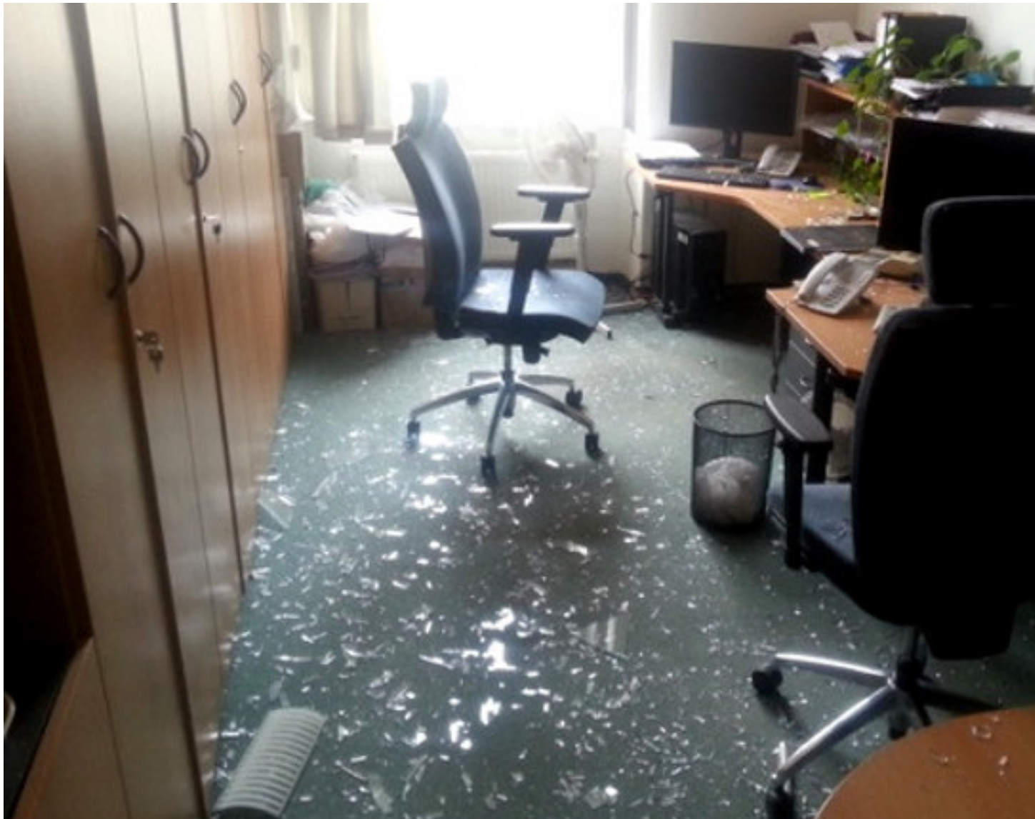
How do things look at the Hollar building a day after the explosion?
